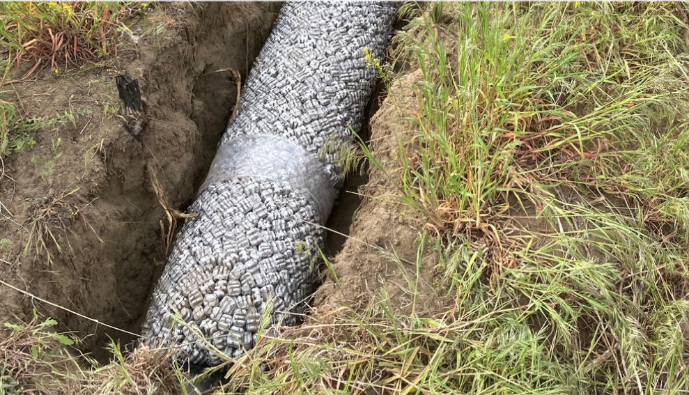
Silver Drainfield - Rocky Flats Campground, WA
