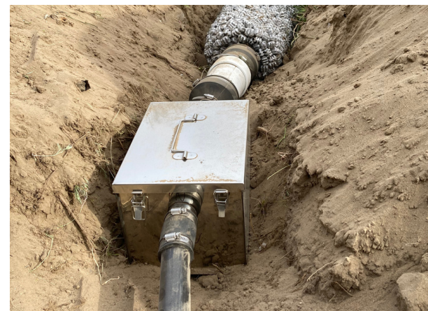
Silver Drainfield - Rocky Flats Campground, WA
